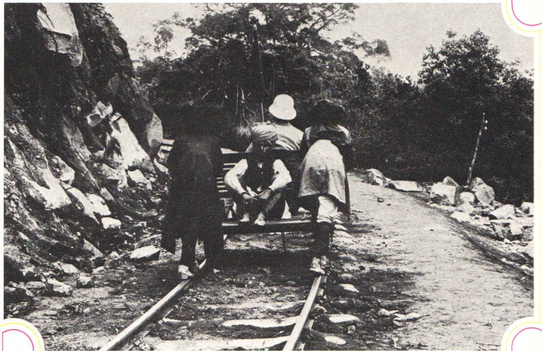
An inspector, sitting on a trolley pushed by coolies over newly laid sections of track, checks that the rails are accurately positioned and firmly secured.
